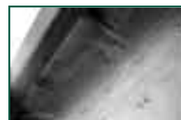
Figure 5: Note the tight seal developed around the roof trusses and the roof-wall juncture.
