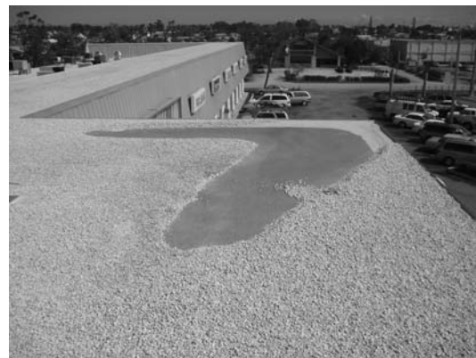
Figure 8: Surface damage (gravel scour).
