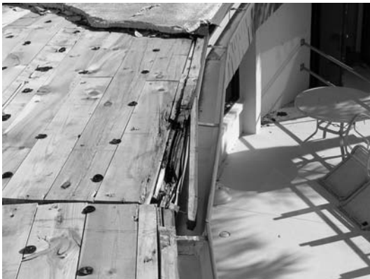
Figure 6: Substrate failure close-up. Edge nailer was rotted and built-up roof was insufficiently fastened.
