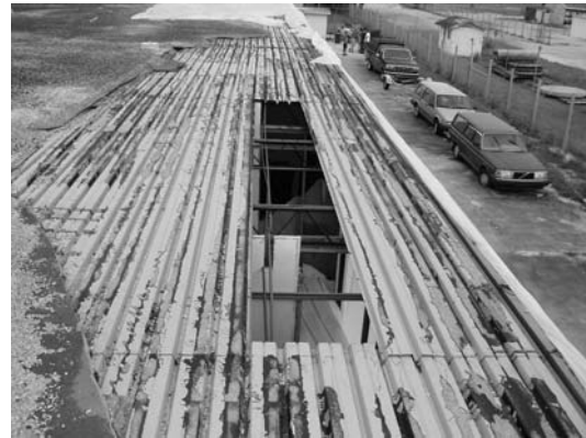
Figure 4: Deck failure. An overhead door failed immediately below the location of this deck failure.
