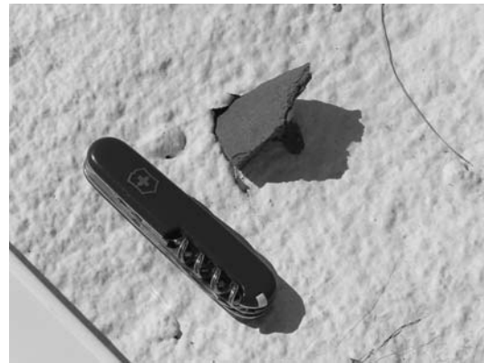
Figure 7: Surface damage (missile impact).
