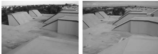
Figure 1: Condominium roof near Jensen Beach. Left photo is before hurricanes Frances and Jeanne. Left photo is after. No damage was observed.
