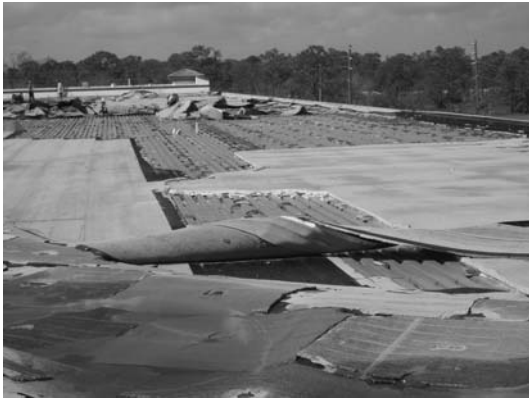
Figure 9: This SPF patch (right-middle of photo) was installed after Hurricane Frances. Hurricane Jeanne damaged the remaining roof, leaving the SPF patch intact.
