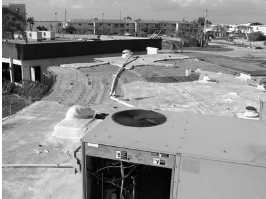
Figure 5: Substrate failure. Deck remained intact, underlying built-up roof peeled up taking SPF recover with it.
