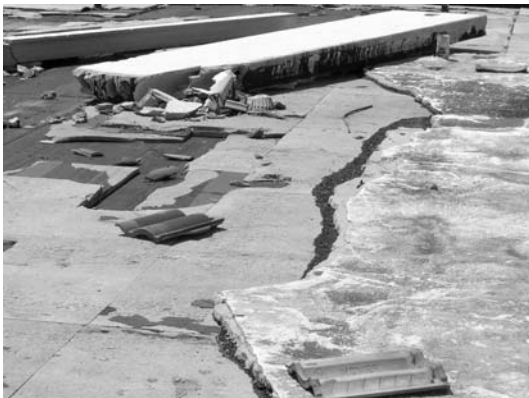
Figure 3: Three modes of failure are evident on this SPF recover of a built-up roof. (1) Deck (hollow-core concrete panels at top); (2) Substrate (built-up roof at left foreground); and (3) Surface Damage (at right foreground).
